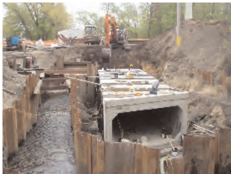
The City replaces the culvert at the mouth of Kids Creek which includes a unique baffle design that provides critical darting cover for younger age-class fish.
